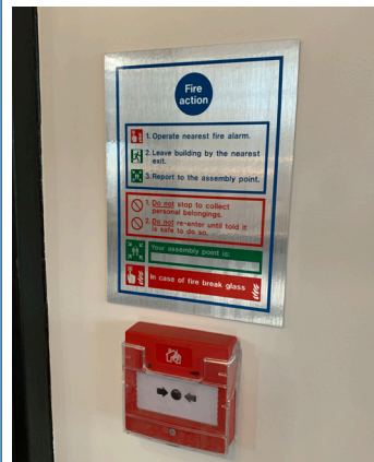
Installation of premium finished signage to customer requirements, not forgetting to install those all-important manual call point covers in some areas to prevent an accidental activation!
