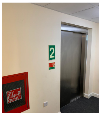
Not forgetting the dry risers being signed correctly on every floor....
