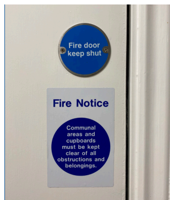
Replacing missing or re-installation of correct mandatory fire door signage.
