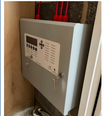
Automatic Opening Vent control panel installation for residential areas for blocks of flats in London
