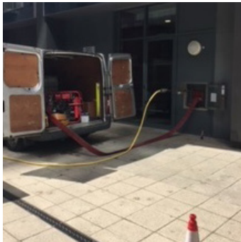
Dry riser inspection and annual wet testing
