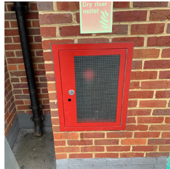
Dry riser remedial works such as replacing glass and fitting compliant signage
