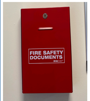
Installation of slimline fire document cabinets in the entrance lobbies of residential blocks of flats
