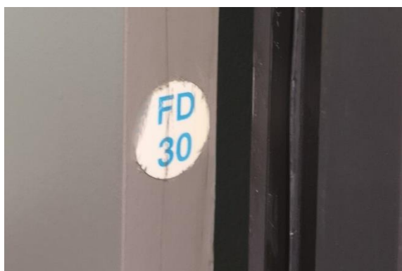
Fire door resistance rating signage
